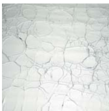
79 113 00 Ixx Cracked Ixx cracked
